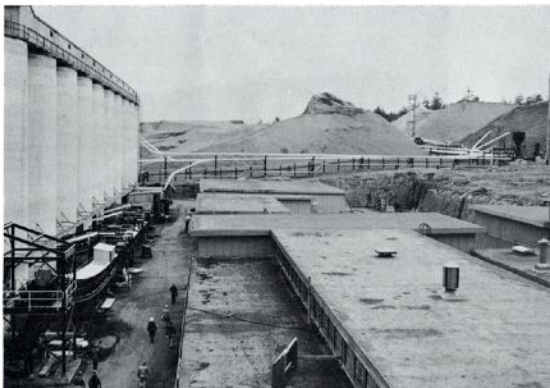
Chip handling system. Chip piles in background with storage silos - left
