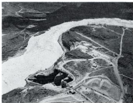
Peace River Dam site. Diversion tunnels through which the water will pass during construction, are seen lower centre.
