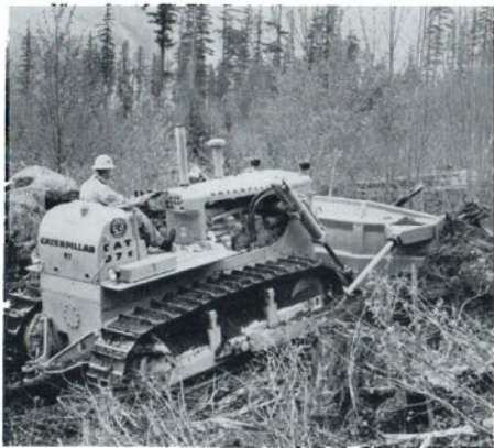
Bulldozers are used to break up the humus layer and expose mineral soil to assure germination of spruce seeds.
