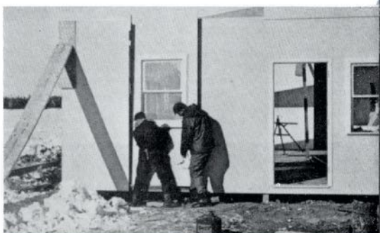
Wall panels almost completed. Interior skin: \frac{3}{8} " G1S Sylvaply; Exterior: \frac{1}{4} " G1S Sylvaply. Both surfaces painted before units shipped.
