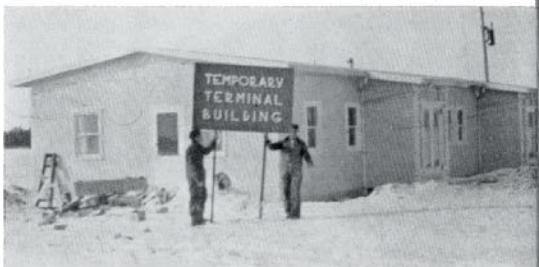
Erection complete. Building is 24'x72' with 8' interior walls. Time: four days. Another five days saw heating installed, floor tile laid, fixtures in, ready for occupancy.
