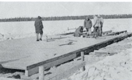
Laying floor panels on joists set right on ground. Interior skin is \frac{3}{8} " Sylvaply Select sheathing grade, exterior skin \frac{5}{16} " Sylvaply Staincote sheathing. Framing: 2"x4" western red cedar.
