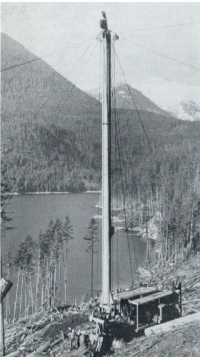
Portable spar quickly erected and in operation. Inset: In portable position for move to new site.
