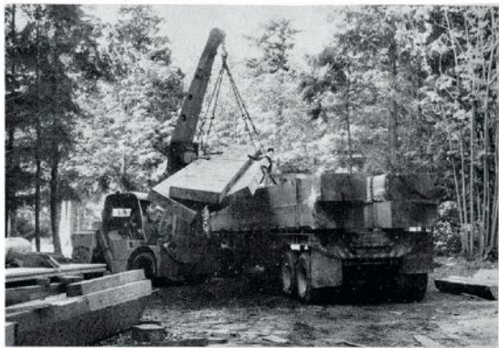
Timbers unloaded at University of British Columbia ready for construction of Long House.
