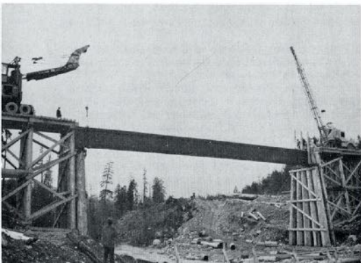
Safe and over, first girder in place. A neat, well done job.
