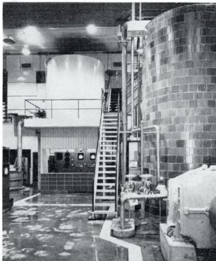
Stock preparation tanks and controls.
