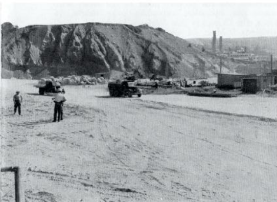
Huge excavation was the first hurdle facing construction crews as work on No. 9 began.
