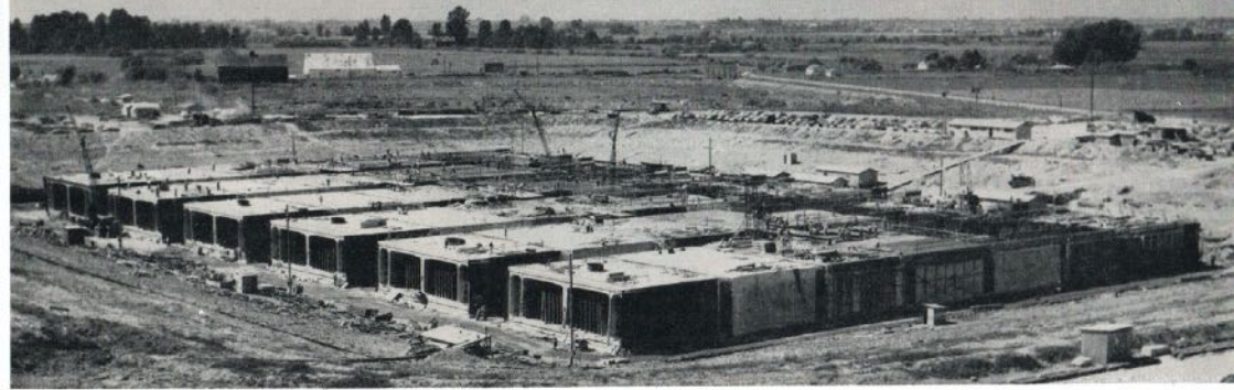
The Deas Island Tunnel sections under construction. When completed they will be floated out to their location in the Fraser River.
