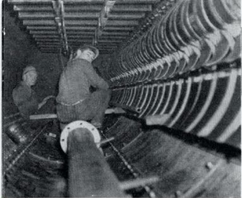
Workmen put finishing touches to the inside of the steam drum for No. 16 Boiler.
