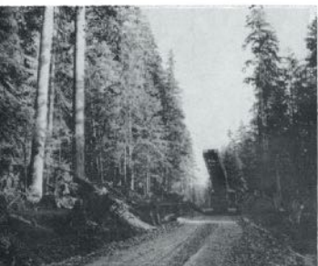
Preliminary Road Has Been Cleared and Shovel With Log-Loading Boom Clears Right-of-Way In Preparation For Widening.
