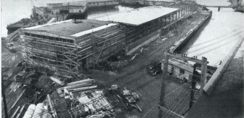
New wharf construction at Powell River showing Administration Building (foreground) and portion of new storage sheds.
