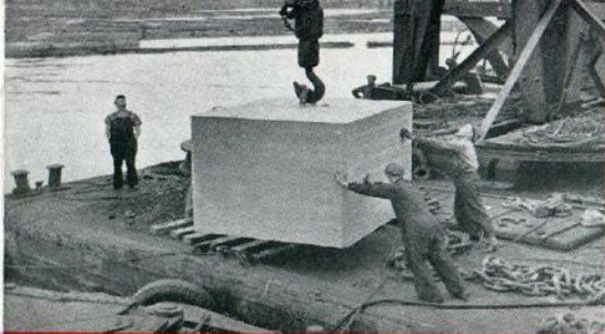
The 16-ton anchor swings off the wharf to the waiting pile driver.
