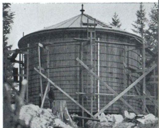
The tank reservoir is situated on a level which guarantees ample water pressure for all residents.
