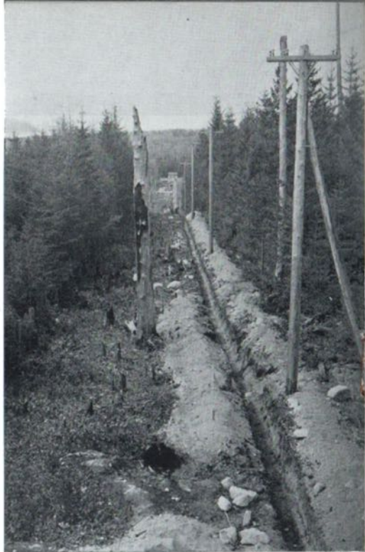
The main feed-line looking from the top of the tank towards Wildwood. The main line reaches the road at DeGroot's Dairy.
