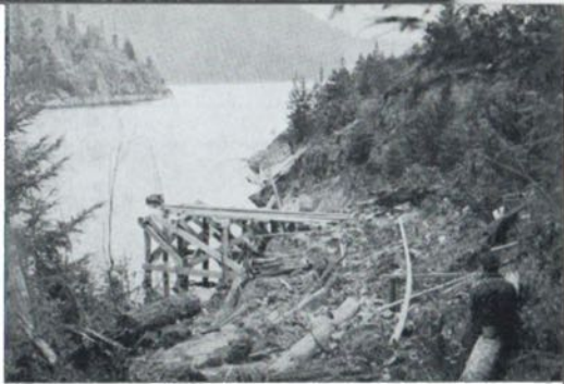
The pipeline reaches the lake. The ramp is ready for installation of the pump expected momentarily.
