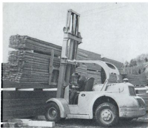
Up we go! No effort at all. Lumber hoisted up and the truck prepares to move off.
