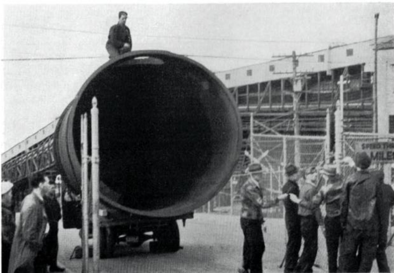
Powell River's Bull Gang in action during an average day. Here, the boys are guiding a new compression chamber for the Sulphite plant through the gates on Second Street.
