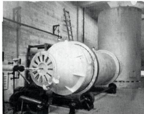
The new sulphite burner and combustion chamber, which replaces the old unit of four burners seen below.
