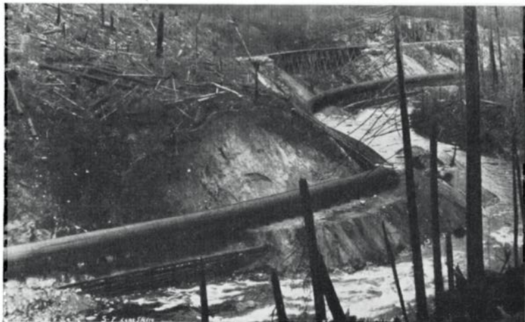
The wood stave pipe line at Lois River winding snake-like along the banks. This line will be eliminated when the new permanent dam is erected.
