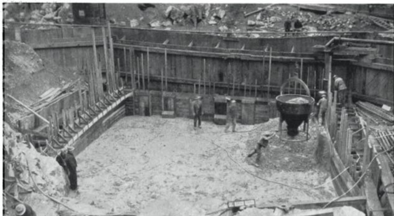
The new dam at Lois River, showing the concrete mixer in action on the dam foundations.
