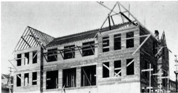
The new Provincial Building at Powell River now in the course of construction. It will be of Tudor design, and an asset to the architectural beauty of the district.
