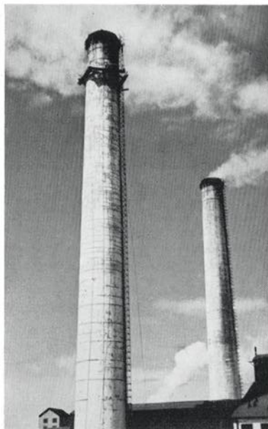
The Steam Plant Stack, showing painters and cleaners at work on its 250-foot sides.
