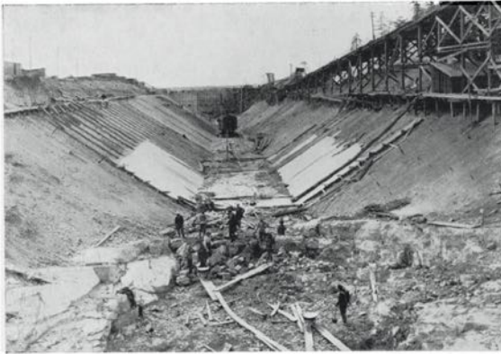
Excavation work on the canal site in 1911. The headgates under construction are seen in the background. The canal was later abandoned and the penstock line run direct from the headgates to the mill.
