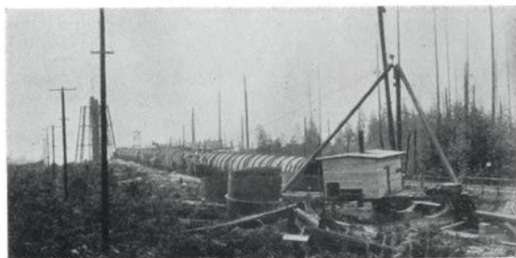
The long 2,700-foot penstock, running from the tunnel entrance to the generator house at Stillwater, crawls like a giant caterpillar over the face of the countryside.
