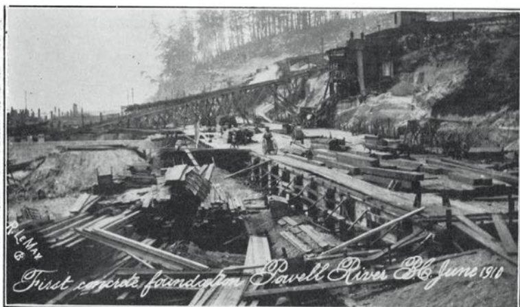
In the summer of June, 1910, mill construction, following the clearing of the townsite, was under way. Above shows the laying of concrete foundations for the "Old" Mill.
