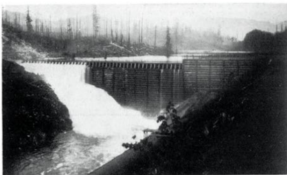
View of the temporary log crib dam at Lois River, which will provide an immediate increase of 22,000 h.p. to our present power capacity. Soon the water will be roaring through the steel penstocks to the power-house at Stillwater.
