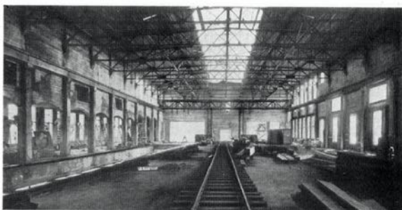
Interior of the new machine room, built to accommodate two 226-inch newsprint machines. Work of installation on the first machine is now under way.
