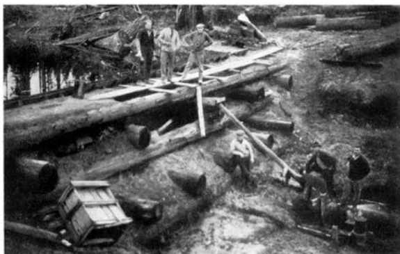
Another view of the dam showing excavation work necessary before the timbers were set.
