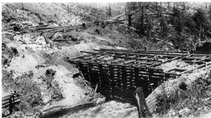
Work on the hydro-electric developments at Lois River is advancing steadily. The temporary log crib dam, to store the initial 22,000 horsepower to be developed immediately, is now well under construction.
