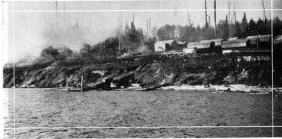
Camp 1, at Stillwater, where Stuart Cameron & Company, contractors, are building the Powell River Company's new power house. Power will be transmitted direct from this site to Powell River.
